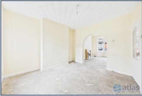
Rear Reception Room
